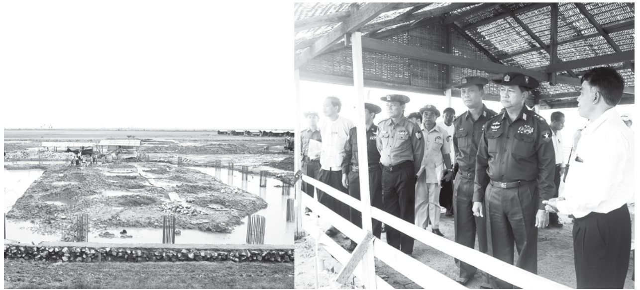
Lt-Gen Ko Ko of the Ministry of Defence inspects construction of cyclone shelter at Thingangyi village in Labutta Township.
