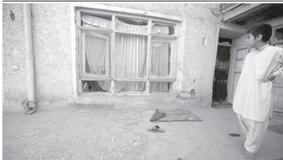
An Afghan boy looks at the broken window of his house after a rocket hit in Kabul, Afghanistan, on 4 Aug, 2009. Five rockets slammed into Kabul at daybreak Tuesday, one of them falling near the US Embassy in a rare attack on the Afghan capital less than three weeks before presidential elections, police and residents said.—INTERNET
