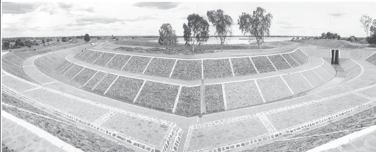
The direct conduit and head regulator under construction at Myaukyama Irrigation System Project in Pale Township, Monywa District.
