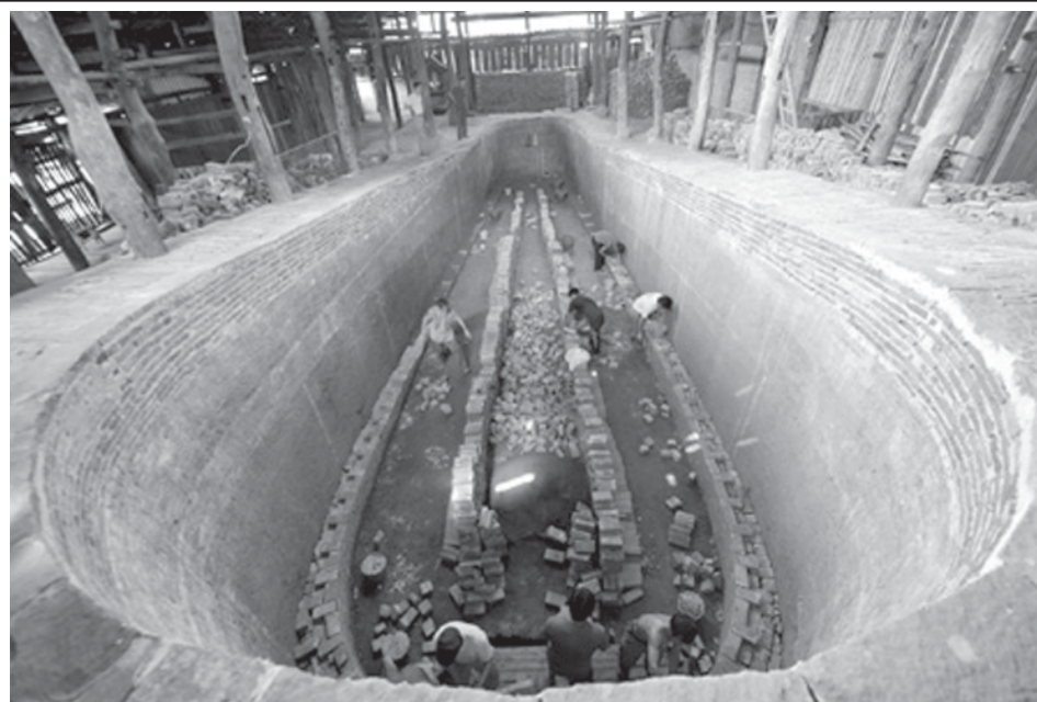
Workers repair an ancient kiln of the Qing Dynasty (1644-1911), in China's porcelain capital, Jingdezhen City, eastern Jiangxi Province, on 1 Aug, 2009.—INTERNET
