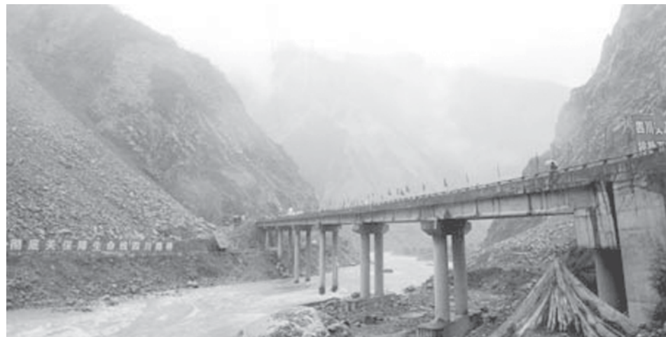
Photo taken on 31 July, 2009 shows the repaired Chediguan Bridge, part of No 213 state highway, in Wenchuan, southwest China's Sichuan Province. The bridge was reopened to traffic on 31 July, seven days after it was damaged by a fallen rock. No 213 state highway is a key traffic line linking Wenchuan County to other areas of Sichuan. —XINHUA
