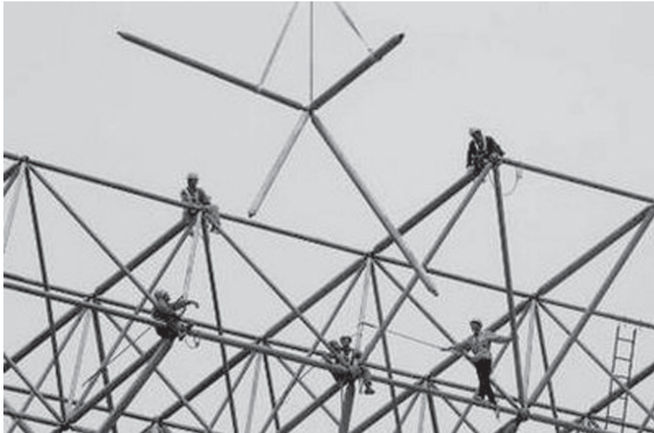
Labourers work on the framework of an unfinished stadium at the construction site in Changzhi, Shanxi Province on 28 July, 2009. —INTERNET
