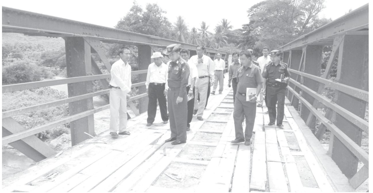
Lt-Gen Min Aung Hlaing views condition of Pyinyaung Bridge on Meiktila-Taunggyi-Kengtung Road.—MNA
