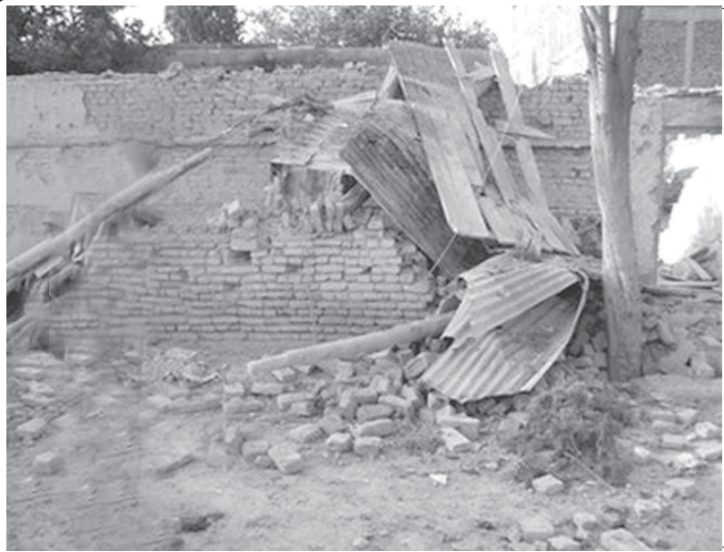
A guard post which was damaged in an attack in Khost, east of Kabul, Afghanistan, on 25 July, 2009. INTERNET
