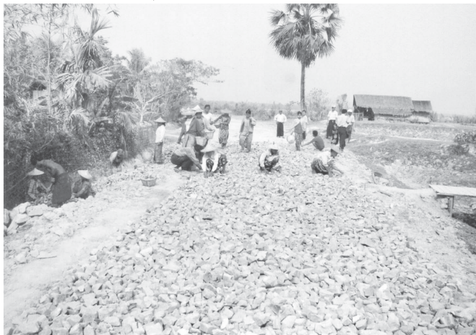
A rural road is being built by Minbya Township Development Affairs Committee.
