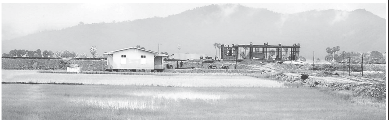
Seikkan station under construction and four-unit staff quarter at Dawei-Thayetchaung railroad section.
