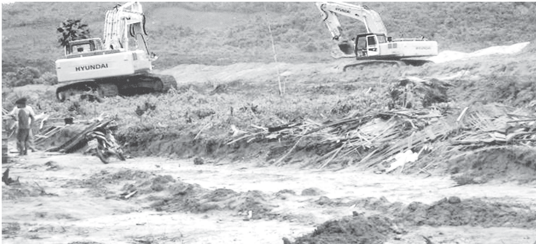
Two excavators at work in Thamok-Bokchan railroad section of Dawei-Myeik Railroad Project.
