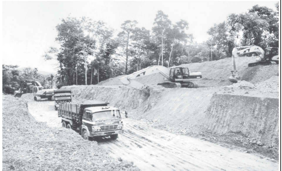
Earthwork in progress at Peindaw in Dawei-Thayetchaung railroad section of Dawei-Myeik Railroad Project.
