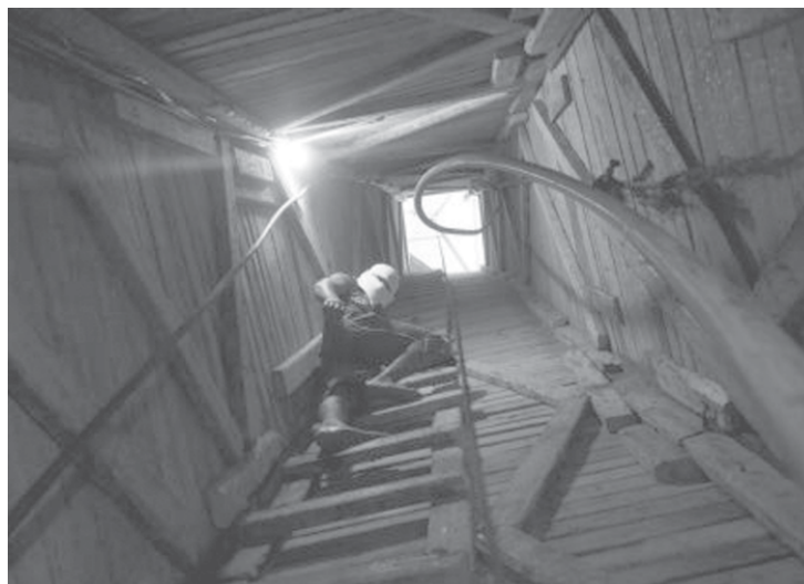
A Palestinian works in a tunnel in Rafah, southern Gaza Strip, on the border with Egypt, on 19 July, 2009. A total of 115 people have been killed in the tunnels in two years.
