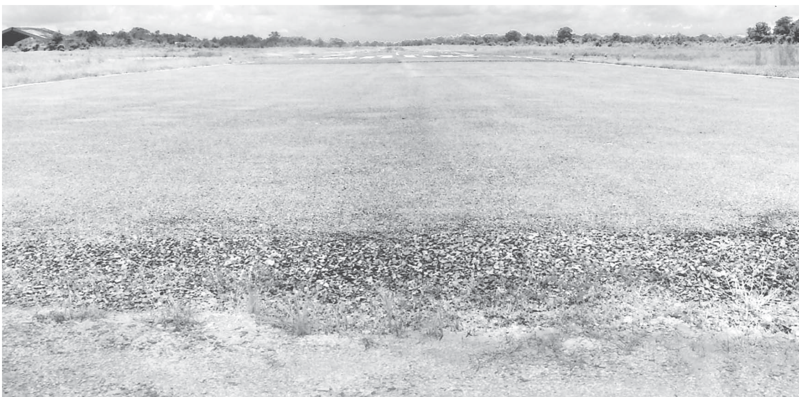
Photo shows the runway of Myitkyina Airport tarmacked by Myitkyina District Public Works.
