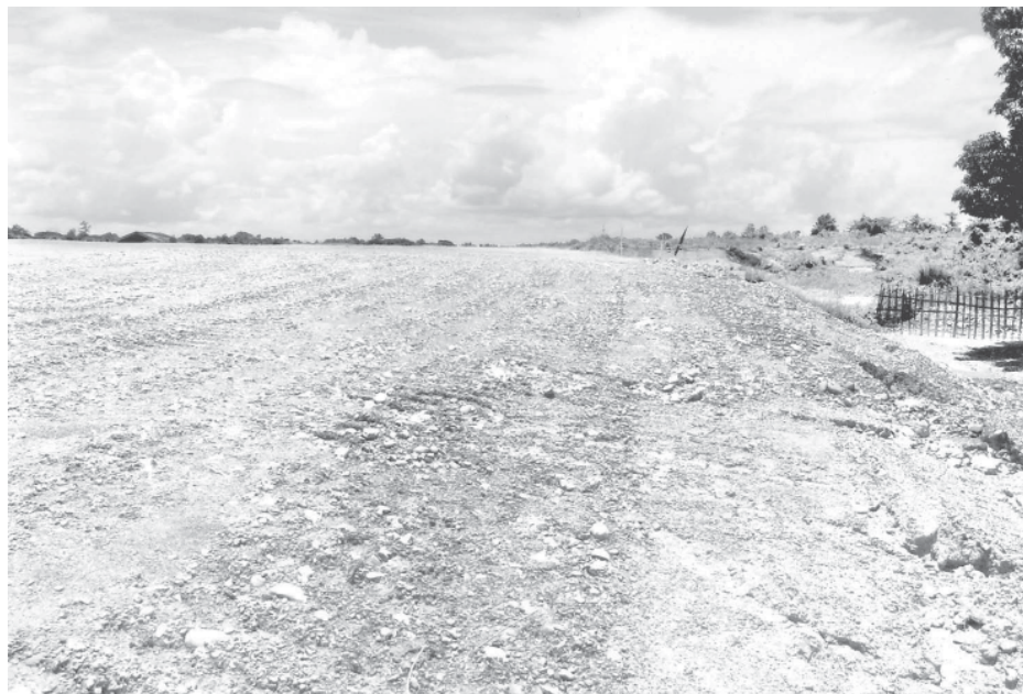
Photo shows progress of ground work on extended runway at Myitkyina Airport.
