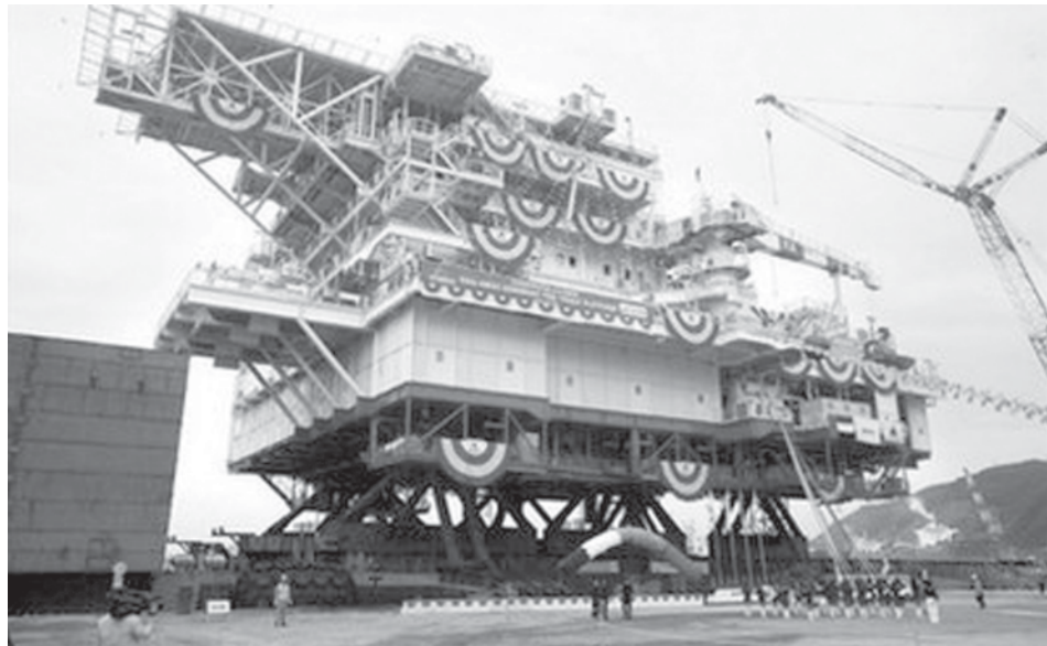
Handout photo shows an offshore oil production platform—destined for the United Arab Emirates—being launched in Ulsan, South Korea. Three firms from South Korea have won orders totalling 3.9 billion dollars for a series of massive gas development projects in the oil-rich region of the Middle East, it has been announced.—INTERNET
