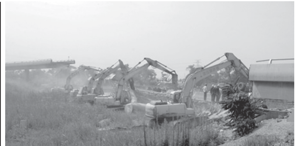
Rescuers clean up the site of the collapsed ramp bridge on the Jinjin Expressway in Tianjin, north China. The accident occurred on early Wednesday morning, when the ramp bridge on the expressway from Tianjin to Shanxi Province suddenly collapsed and five vans crashed, causing six people dead and four others injured. The investigation of the accident was underway.—INTERNET
