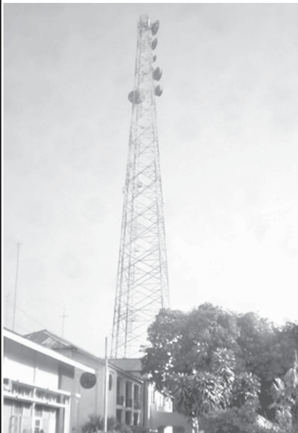
A microwave tower seen at auto-exchange in Sittway.
