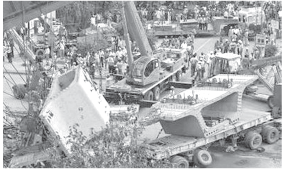
A rescue operation is in progress after a Delhi Metro Rail Corporation (DMRC) flyover collapsed in New Delhi on 12 July, 2009. At least five people are feared to be dead and several others injured after a part of the flyover which was under construction collapsed on Sunday, local media reported.—INTERNET
