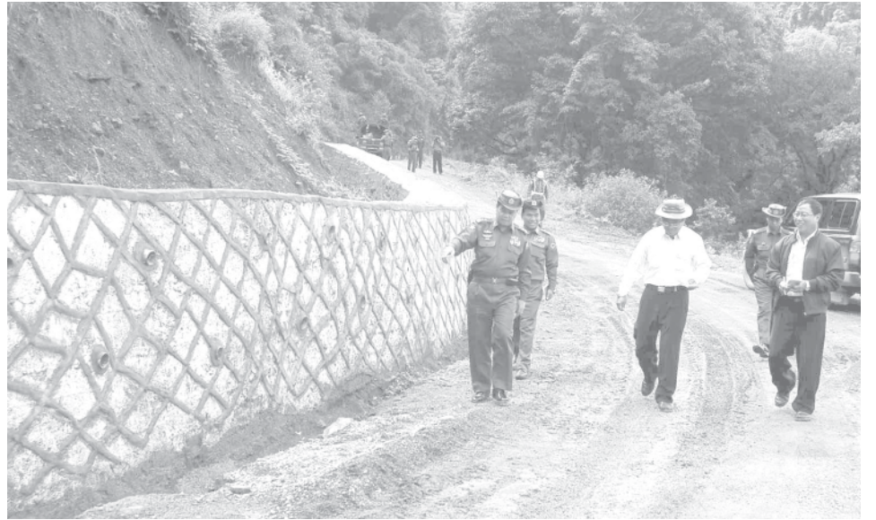
Lt-Gen Tha Aye of Ministry of Defence inspects gravel retaining wall of Mindat-Matupi Road and extended construction of road.—MNA
