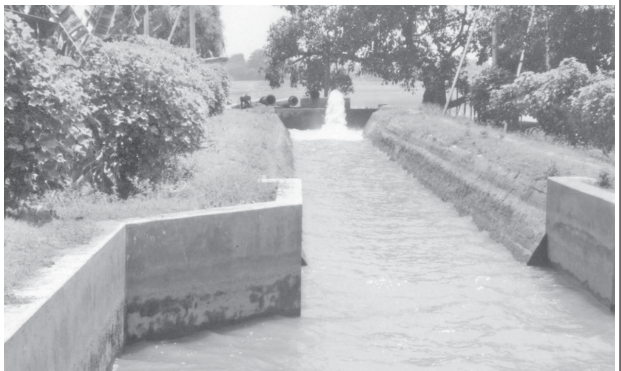
Water is pumped from Chindwin River into the main canal to irrigate farmlands.
