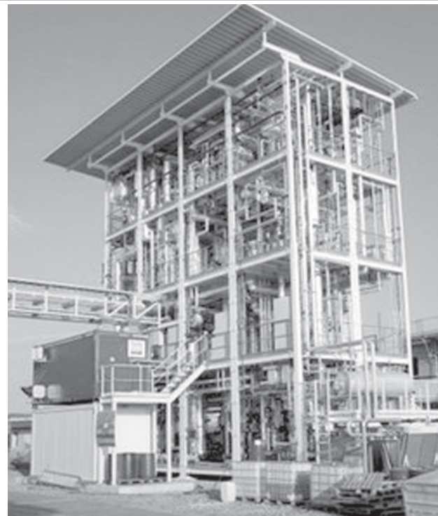
The exterior of a new European Center for Renewable Energy plant that produces gas from wood in Guessing, southeastern Austria, paving the way toward new possibilities in renewable energy. The facility in Guessing, a town renowned for being entirely energy self-reliant, can produce some 100 cubic metres of bio-gas per hour.—INTERNET
