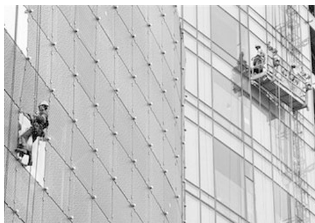
Workers hang off the facade of a new mall at Singapore's major shopping district on Friday July 3, 2009. The Singapore government expects its economy to shrink up to 9 percent this year, the worst recession since independence from Malaysia in 1965.
