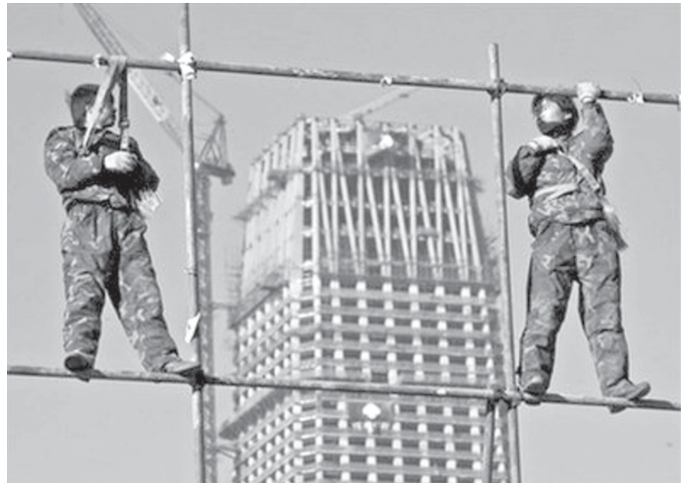
Two Chinese workers erect scaffolding in Beijing's Central Business District. China is weighing a plan to set up a new company to manage some of the country's nearly 18 trillion yuan (2.6 billion dollars) in state assets, a report has said.—INTERNET
