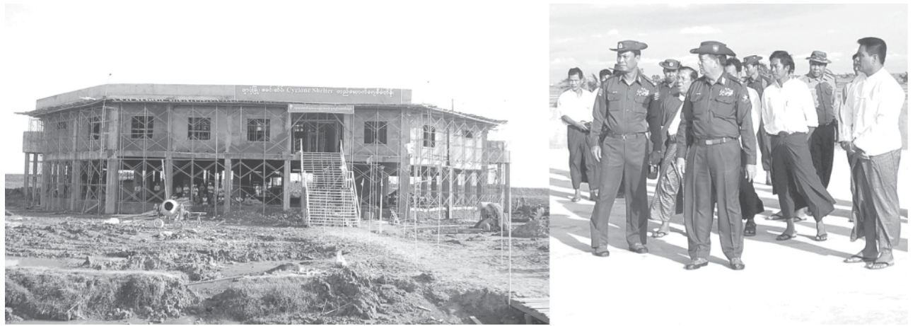
Maj-Gen Ko Ko views construction of Cyclone Shelter in Damiseik Village of Pyapon Township. —MNA
