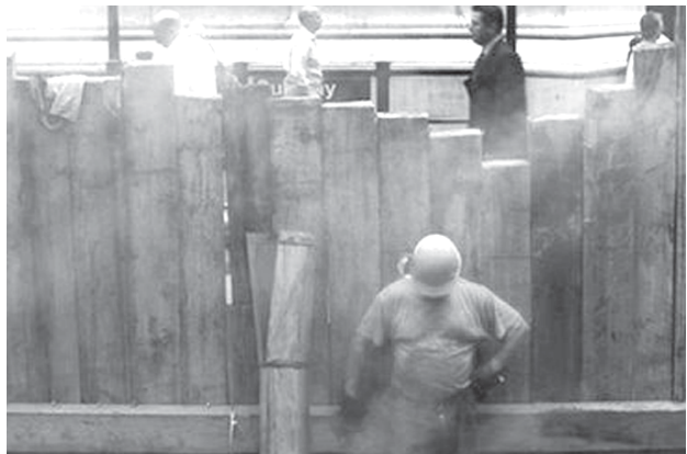
Construction work on Wall Street in front of the New York Stock Exchange. A jittery bond market and economic "green shoots" notwithstanding, the Federal Reserve is likely to reaffirm a commitment to keep pumping money into the economy to battle recession, analysts say.—XINHUA
