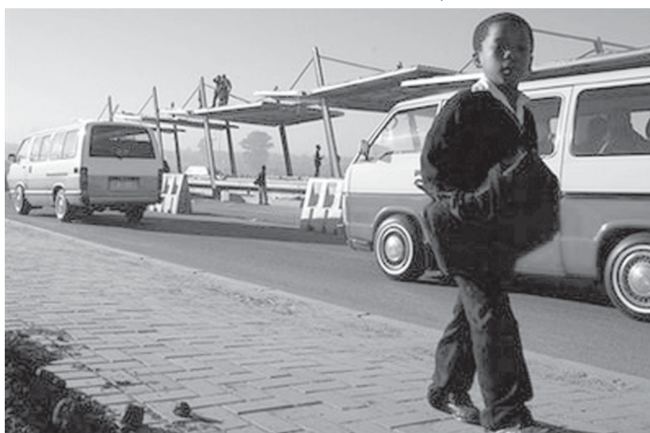
A mini-bus station is seen under construction in Soweto. Pretoria and Johannesburg are each hosting Confed matches, but the two cities lie 60 kilometres (35 miles) apart and are linked only by a traffic-clogged highway that regularly turns the trip into a drawn-out journey.—INTERNET
