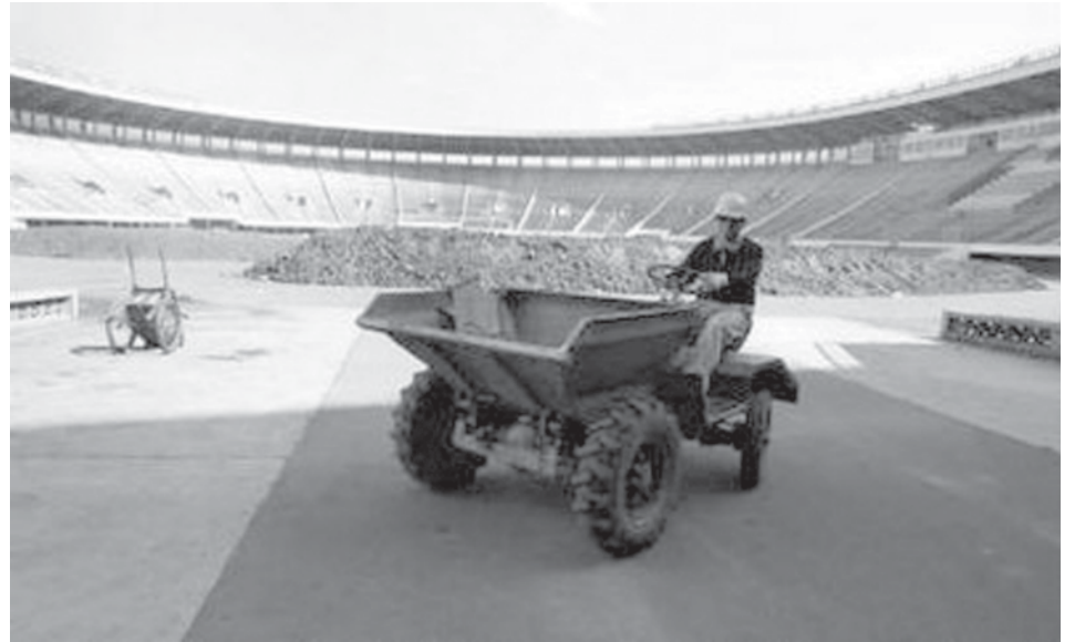
A labourer works at the Zimbabwe National sports stadium in Harare, on 17 June, 2009. The 60,000 seater stadium is currently under renovations in preparation for the soccer World Cup 2010 to be held in neighbouring South Africa in June next year.—INTERNET
