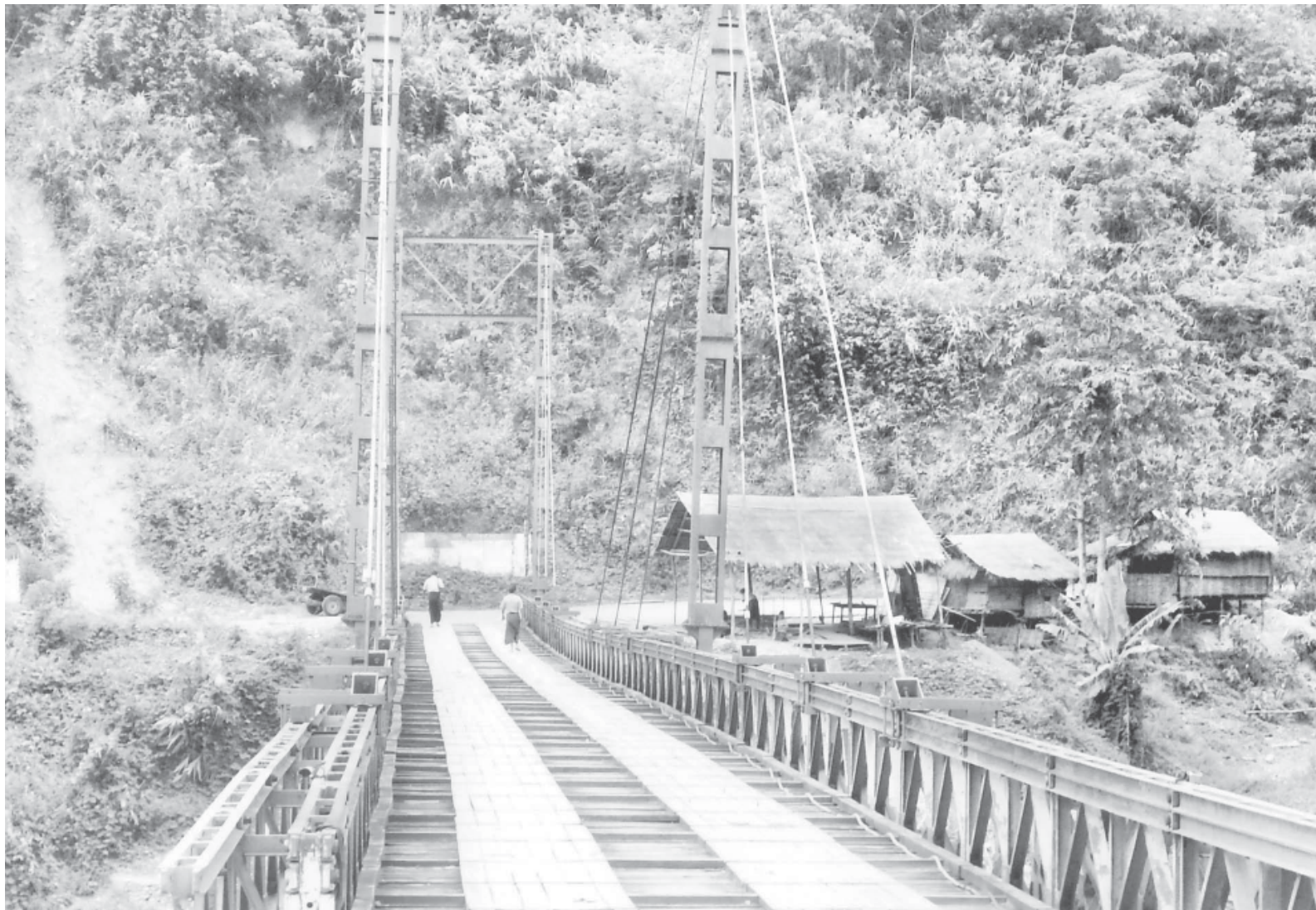
Lelu Bridge linking Namsang Township and Namtu Township in Shan State (North).
