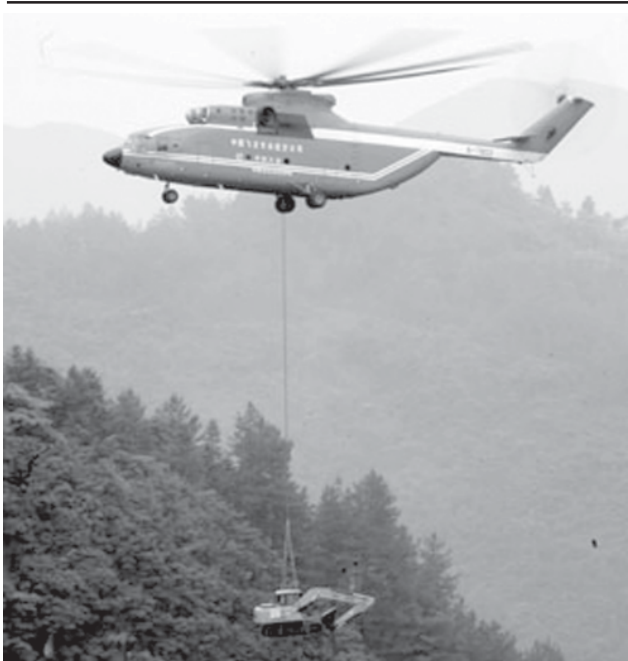
A MI-26 helicopter carries an excavator to the landslide site of Jiwei Mountain, in Wulong County, southwest China's Chongqing Municipality, on 11 June, 2009. The MI-26 heavy-lifting helicopter has begun carrying heavy machineries needed in the search for 63 people missing in a massive landslide on Friday.—XINHUA
