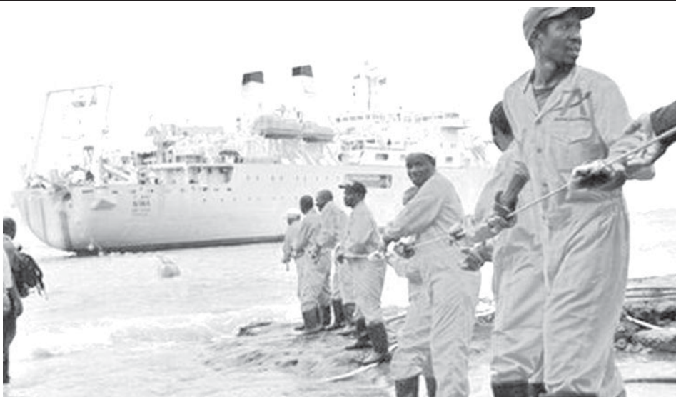
Workers haul part of a fibre optic cable onto the shore at the Kenyan port town of Mombasa. An undersea fibre optic cable bringing broadband Internet connectivity to east Africa, reached the Kenyan coast from the United Arab Emirates on Friday, the president said.—INTERNET
