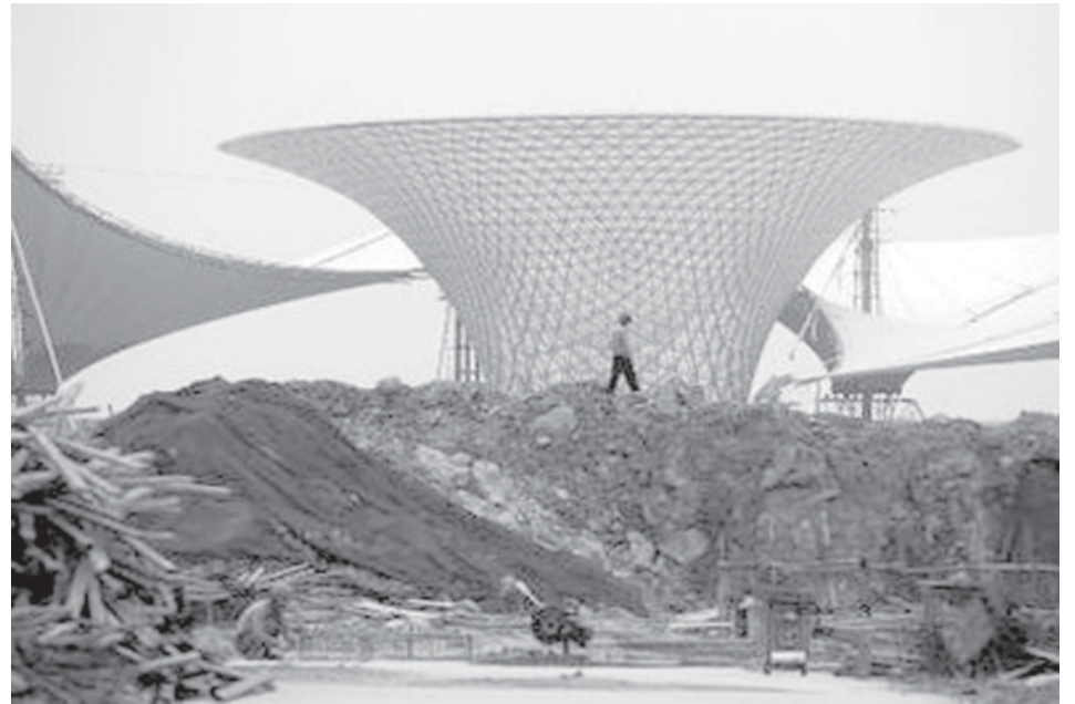
A worker walks in front of a special solar energy construction at the Shanghai 2010 Expo site in Shanghai on 8 June, 2009. —INTERNET
