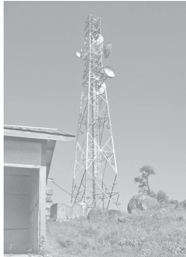
Photo shows a microwave station in Mongpyin.
