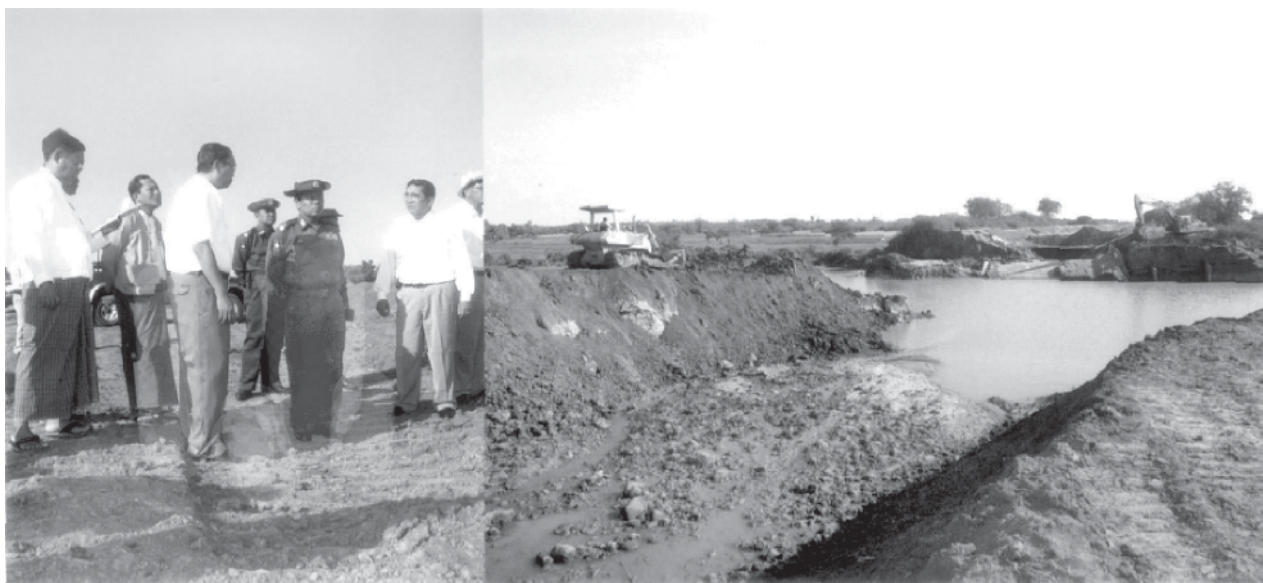
Commander Maj-Gen Tin Ngwe inspects repair of left canal of Kinda Dam in Myittha Township.—MNA
