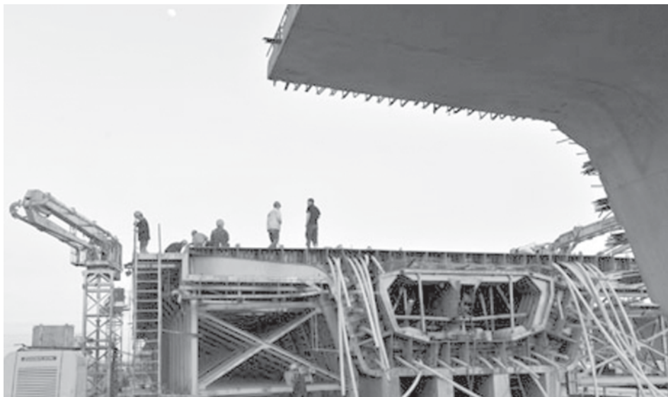
Workers weld a section of steel case beam in Qingdao, a port city in east China's Shandong Province, on 2 June, 2009.—XINHUA
