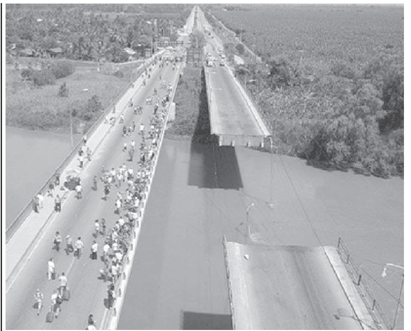
One of the lanes of 'La Democracia' bridge over the Uluá river, built by the French in 1963, had its central section collapse due to an earthquake in El Progreso, 270 km north of Tegucigalpa. A powerful 7.1-magnitude earthquake rocked the economic and tourist heart of Honduras, killing five, wounding at least 13, and shaking neighboring countries as far away as Mexico.—INTERNET
