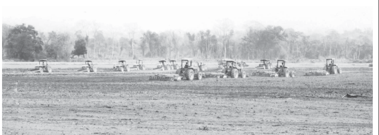
Land preparations being made with the use of heavy machinery at Yuzana Integrated Farm Project.
