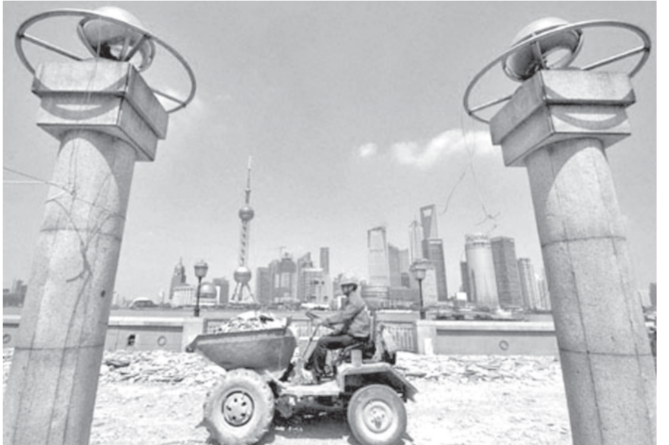
A man works at the construction site along the riverside of the Bund in Shanghai, China, on 26 May, 2009. The reconstruction project of the riverside along the Bund in Shanghai started recently. —INTERNET
