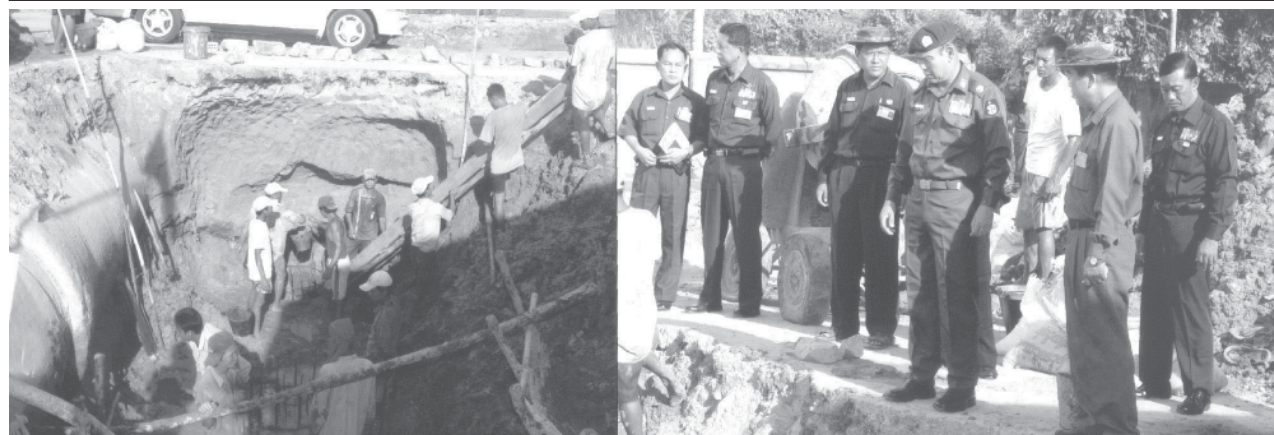
Yangon City Development Committee Chairman Mayor Brig-Gen Aung Thein Lin inspects construction of box culvert for Thamaing Creek across Baho Road between Hline and Mayangon Townships.—MNA
