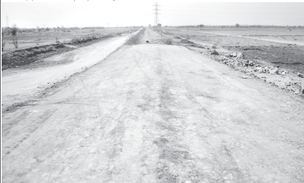
A road section of Inter-District Road (2), about 10 miles to east of Thazi.
