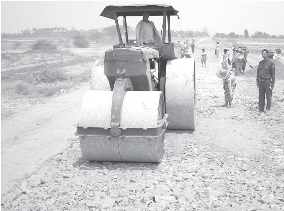
Gravel road section at mile post No. 100/4 of Inter-District Road (2) in Thazi Township.
