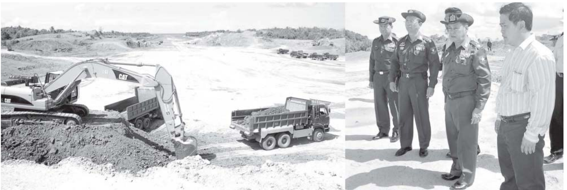
Prime Minister General Thein Sein inspects progress of Thandwe airport runway extension project.—MNA
