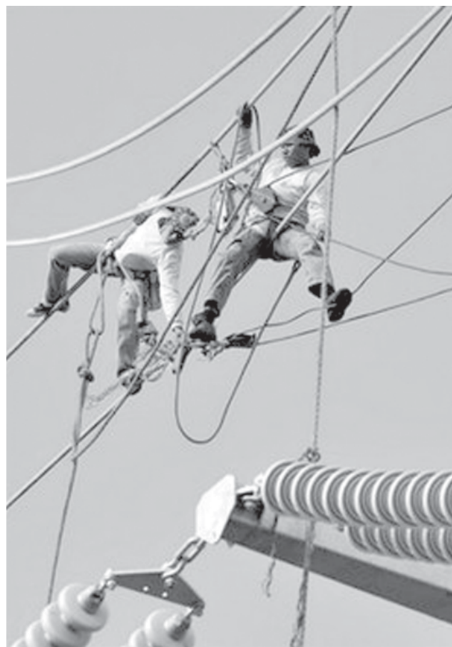
Filipino linemen install cables in Santa Rosa, near Manila in early January. A billion-dollar bond offering by the Philippines state agency which runs National Power was nearly six times subscribed, the government and reports have said.—XINHUA
