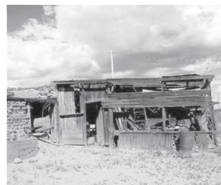
This undated photo provided by Josh Bond shows the old stable from the days that the Old Cuchillo Bar was a busy stagecoach stop in Cuchillo, NM. Owner Josh Bond has invited the West Coast Ghost and Paranormal Society to investigate strange noises and falling objects on the 180-year-old property.
