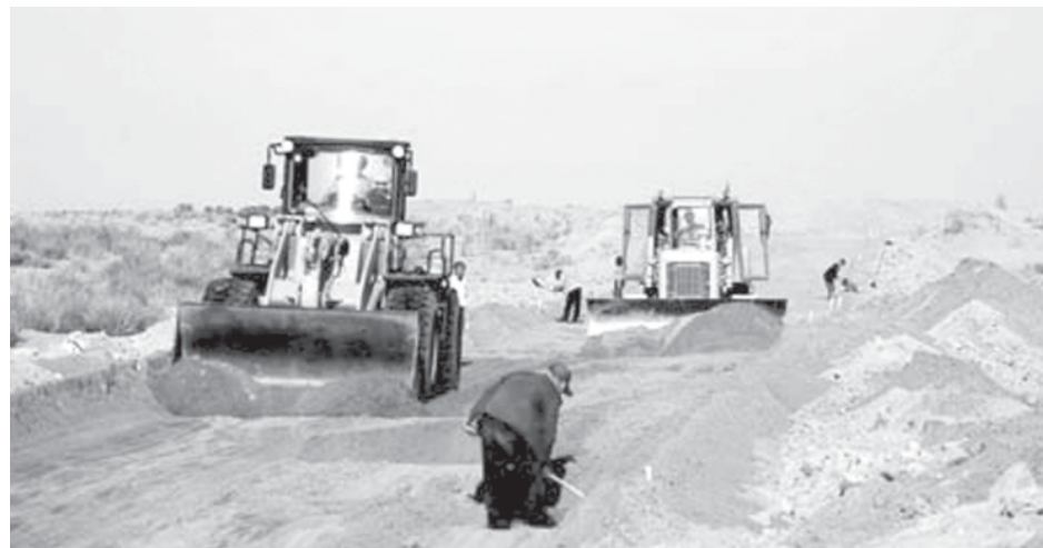
People manipulate bulldozers to work in Ulan Buh Desert of north China's Inner Mongolia Autonomous Region, on 12 May, 2009. China starts to build the first road through the desert recently. With the length of 71.6 kilometres, the road will be put into use on 30 September. XINHUA
