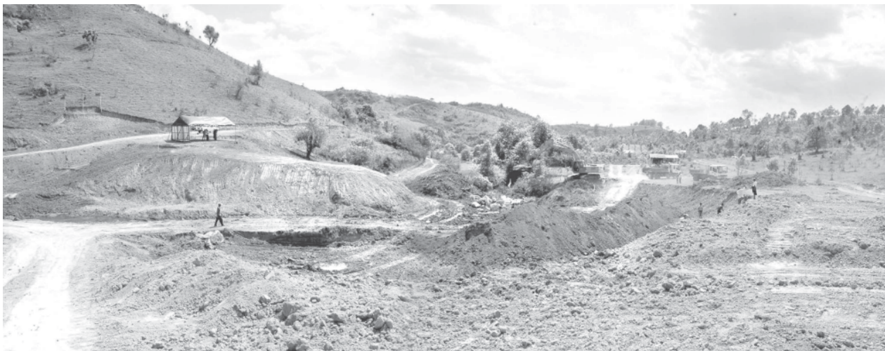
Land preparations being made for construction of Htithein Water Supporting Dam near Taunggyi.
