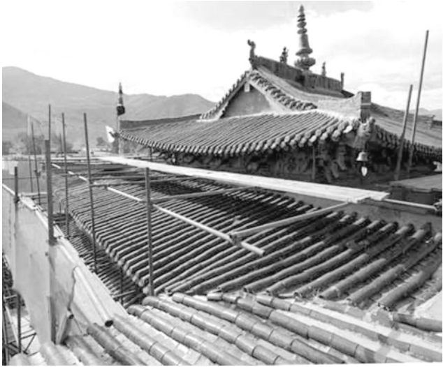
The picture taken on 13 May, 2009 shows some scaffoldings put up at the Shalu Monastery in Xigaze, southwest China's Tibet Autonomous Region. The reparation of the monastery was started on Wednesday. It is planned that more than 16 million RMB yuan will be put on the reparation of the old monastery, which was built in 1027.—INTERNET
