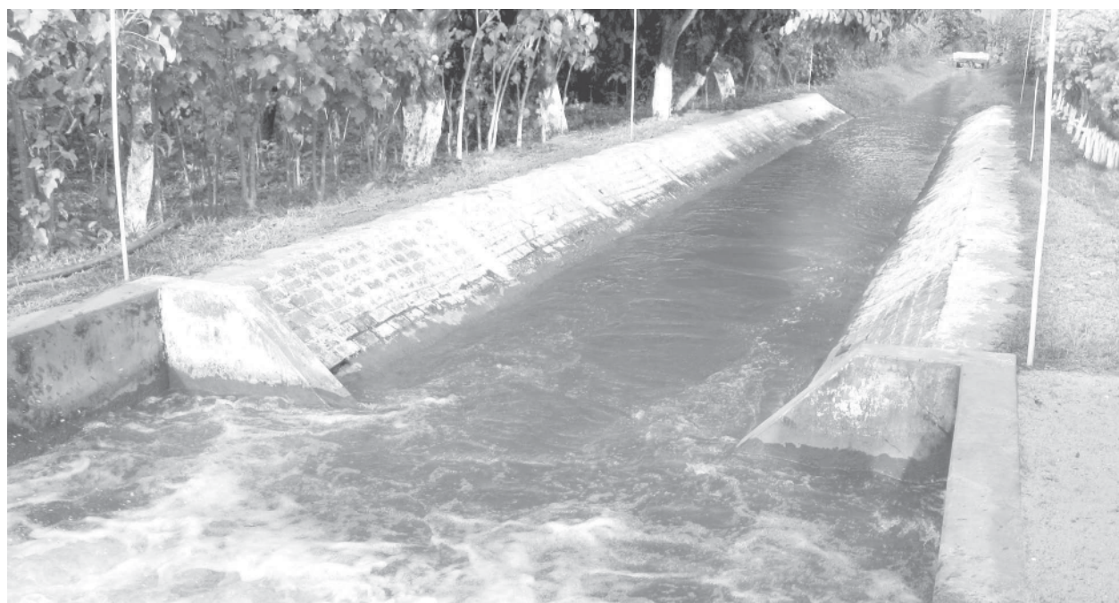
Water flows into the main canal of Tayokhla River Water Pumping Station.
