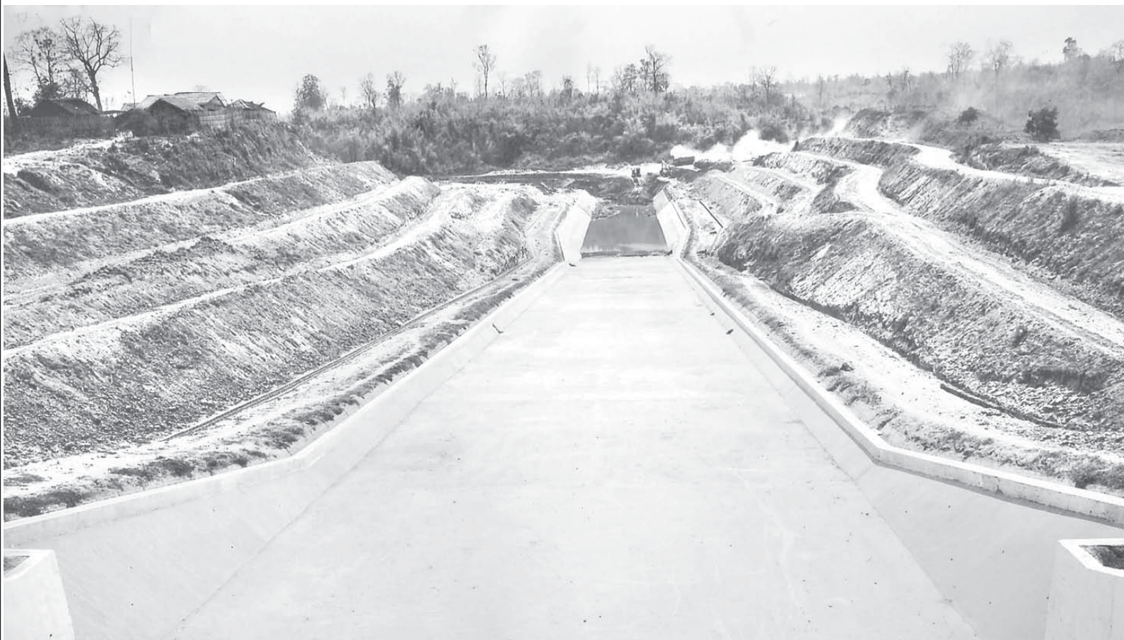
The 790 feet long and 50 feet wide spillway under construction of Madan Dam.
