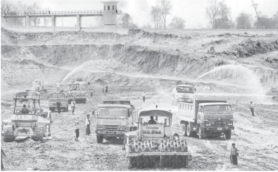
Groundwork is being carried out at a construction site of Madan Dam Project in Nay Pyi Taw Lewe.
