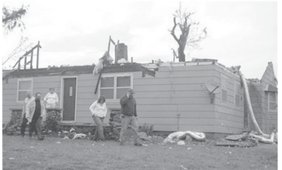
Friends and family members of Jim and Marsha Beggs try to contact them after inspecting damage of their home north of Carl Junction, Mo, which was hit by high winds on Friday morning, on 8 May, 2009. Many cities in southwest Missouri were without power after severe thunderstorms rocked the area.—INTERNET
