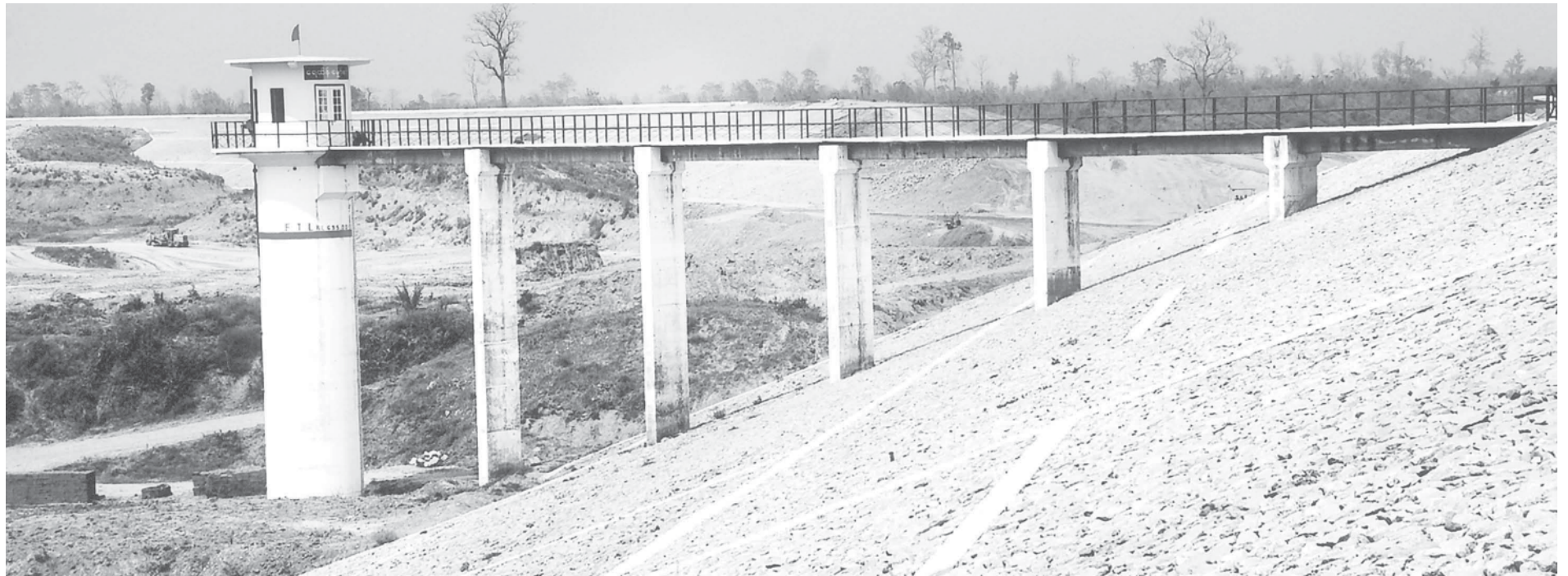
The control tower under construction of Madan Dam near Nanwin Village, Nay Pyi Taw Lewe.
