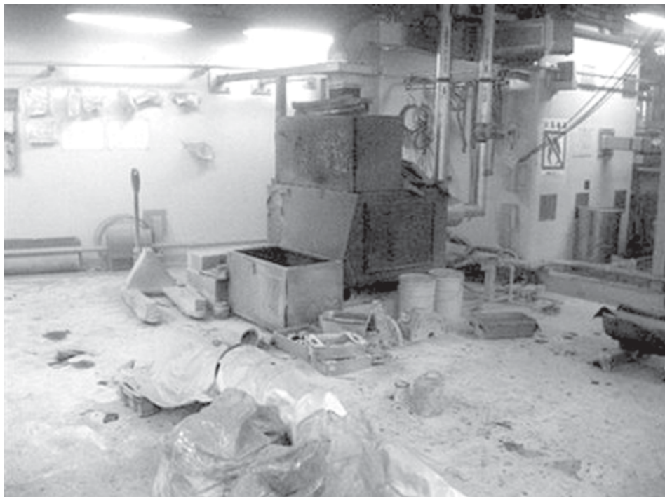
A pump room at the suspended reactor of the Kashiwazaki-Kariwa nuclear plant, in Kashiwazaki, about 225 kilometres northwest of Tokyo, after a small fire was extinguished at the plant.—INTERNET
