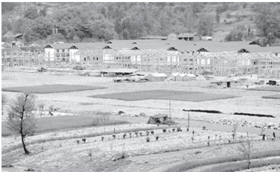
New houses are under construction in Qingchuan county, southwest China's Sichuan Province on 6 May, 2009.
