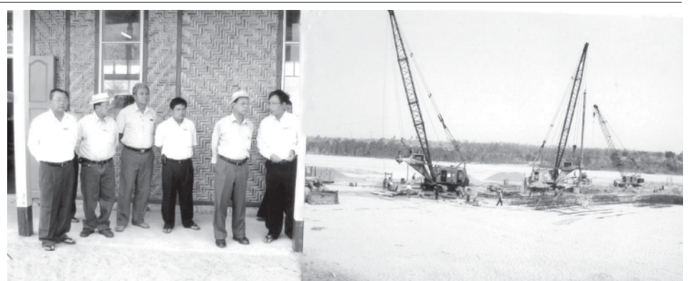
Deputy Minister for Construction U Tint Swe inspects construction of Daungnyachaung Bridge on Yangon-Pyay-Magway-Mandalay Highway.—MNA
