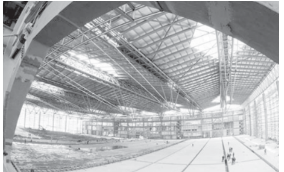
Construction workers get along with the interior decoration inside the west exhibition hall of the Theme Pavilion for the Shanghai 2010 World Expo, in Shanghai, east China, on 26 April, 2009. The west exhibition hall of the Theme Pavilion for the Shanghai 2010 World Expo, extending to 180 meters from north to south and 126 meters from east to west, is noted for a distinguished architectural structure free of pillars, the largest of its kind in China.—INTERNET
