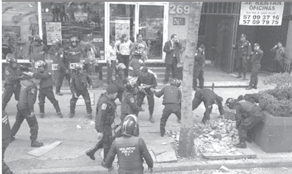
Mexican policemen remove rubble from a building where an auditorium inside collapsed in Mexico City on 23 April, 2009. At least 13 people were injured in Mexico City on Thursday when the roof of a concert hall collapsed in the central neighbourhood of Roma, the city's Civil Protection Department said.—XINHUA
