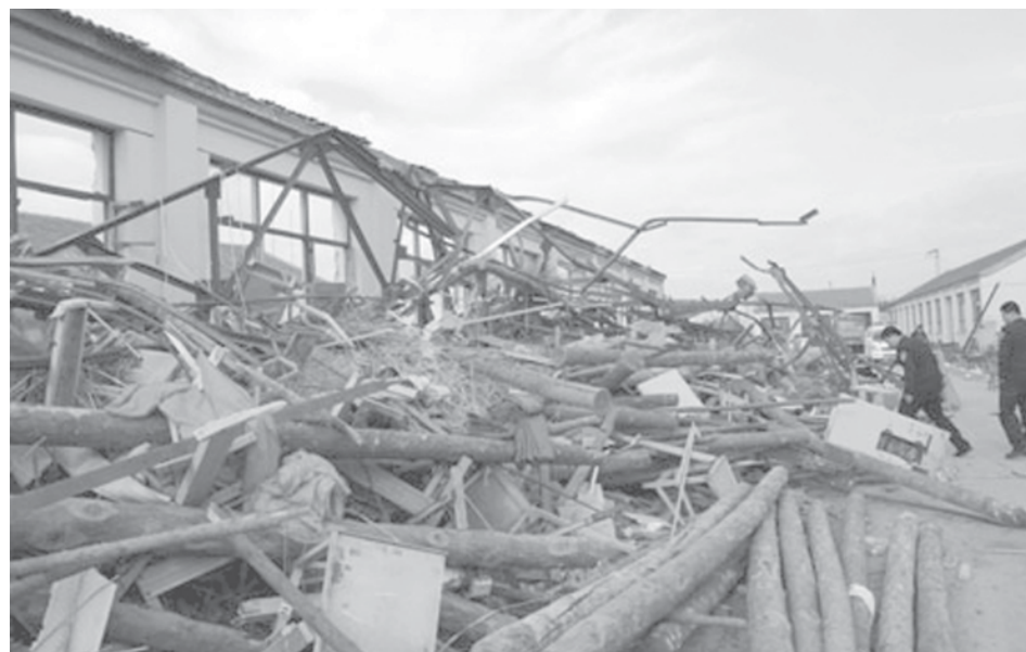
Workers collect articles at the site of roof collapse in Langfang, a city in north China's Hebei Province, on 24 April, 2009. At least 10 people were killed and 15 others injured after the roof of a clothing factory collapsed in Langfang on Friday. —INTERNET
