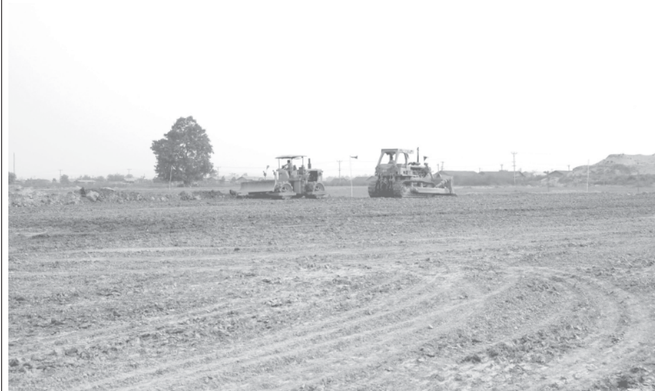
Land preparations being carried out at the site for main building of Nay Pyi Taw International Airport with the use of heavy machinery.
