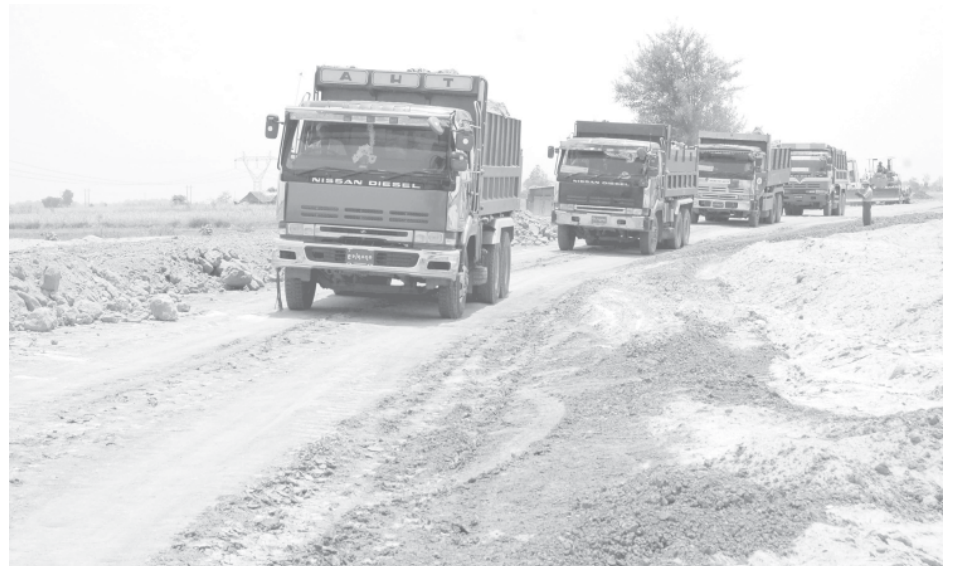
Groundwork being undertaken at first phase construction of buildings for Nay Pyi Taw International Airport with the use of dumpers.—MNA
