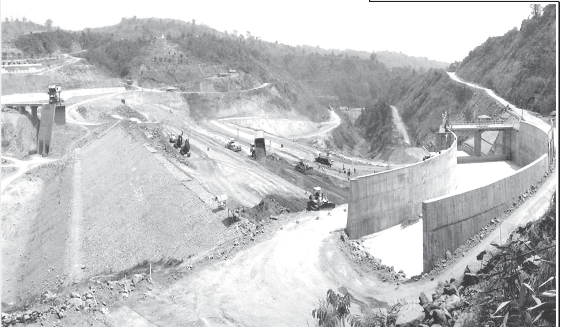
Main embankment and spillway (water intake canal) are under construction in Kunchaung Hydropower Project in Pyu Township of Bago Division.
