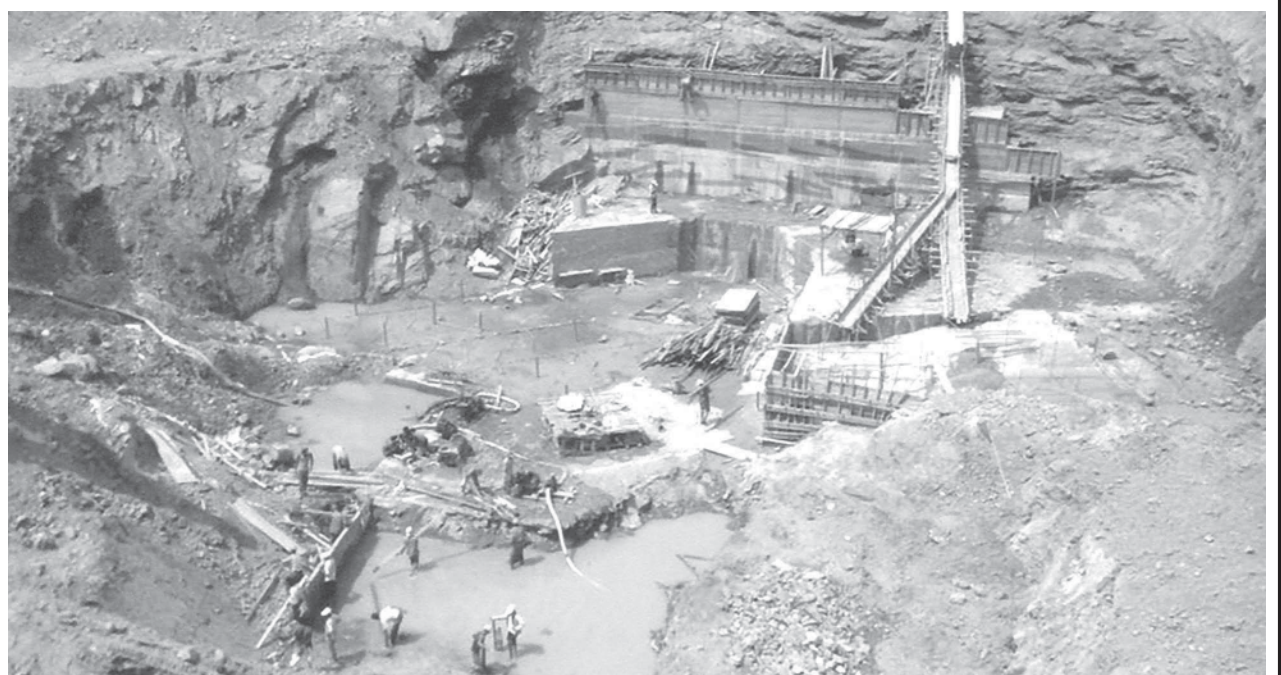
Land preparation has completed by 29 per cent for construction of power plant on 31 March.
