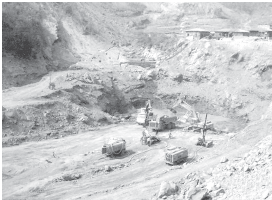
Land preparation being made with the use of heavy machinery for building Power Plant of Pyuchaung Hydropower Project on 30 March.
