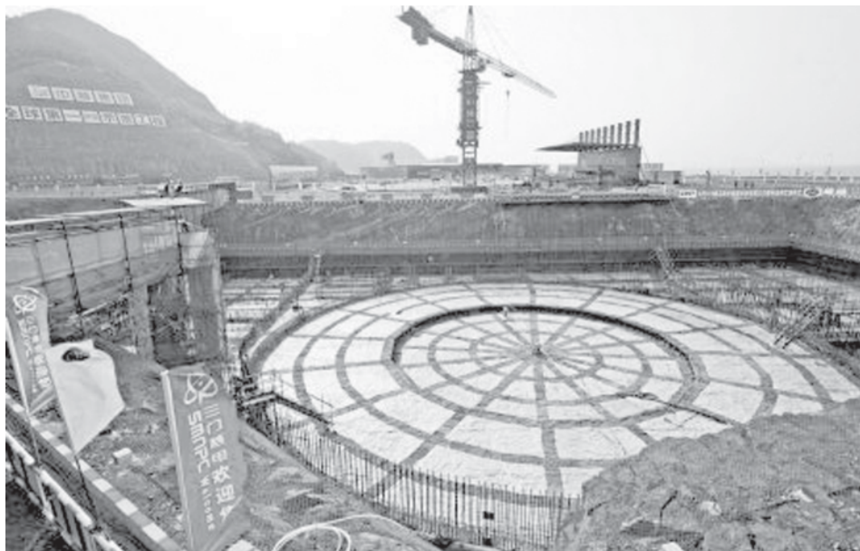
Photo taken on 18 April, 2009 shows the foundational construction site of the No 1 unit of the first phase of the Sanmen nuclear plant in Zhejiang Province. The Sanmen nuclear plant, with the world's first nuclear plant using the AP1000 technologies, a type of third generation nuclear power reactor introduced by America's Westinghouse company, started the construction recently. —XINHUA
