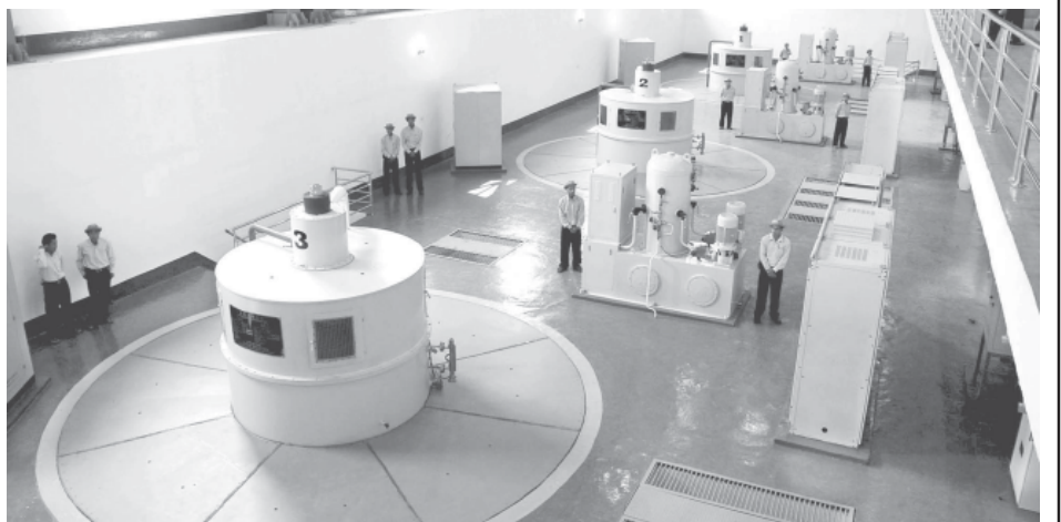
Three vertical-type Francis generators installed at Kengtawng Hydropower Plant.
