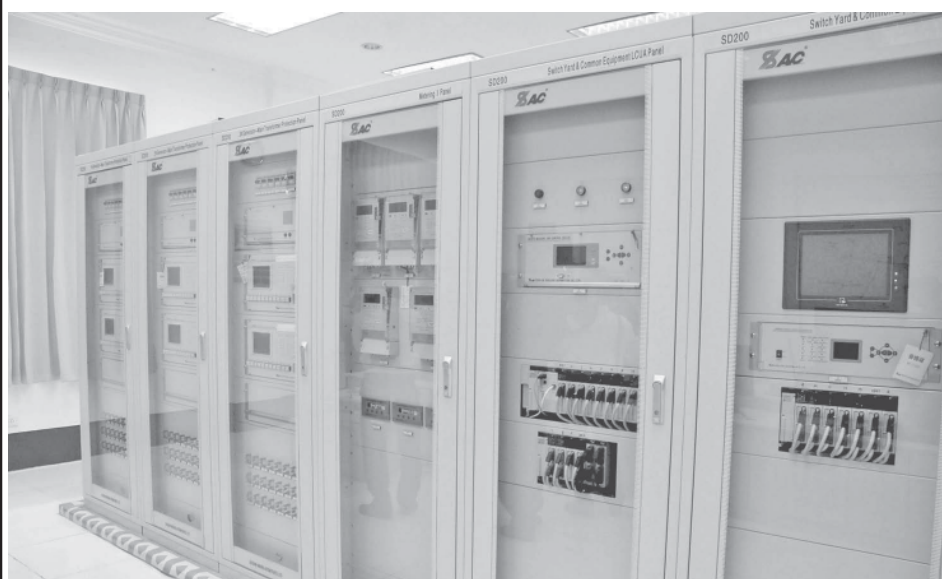
Modern equipment installed at central control room of Kengtawng Hydropower Plant.
