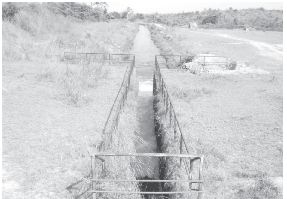
Photo shows supply of water from Bawni Dam through a canal in DaikU Township.
