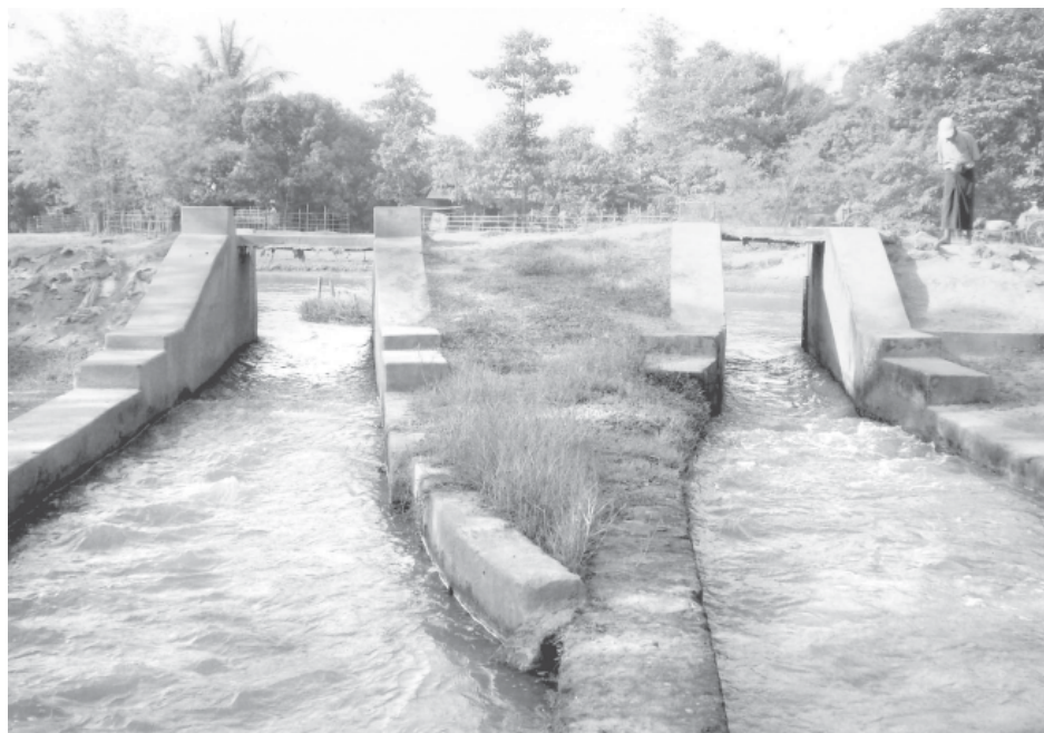
Water being supplied from Bawni Dam to Tabinshwehti Sluice Gate in Kadokywama Village.
