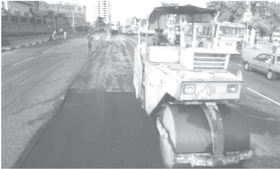
Major road maintenance near 8th mile junction in Mayangon Township in progress.—MNA
