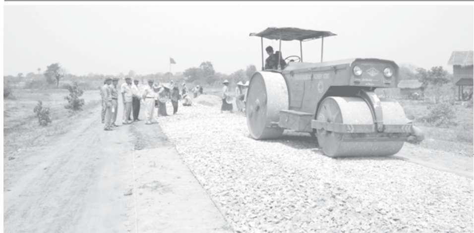
Director-General of Development Affairs Department U Myo Myint inspects progress in construction of No. 2 inter-district road in Mandalay.—PBANRDA
