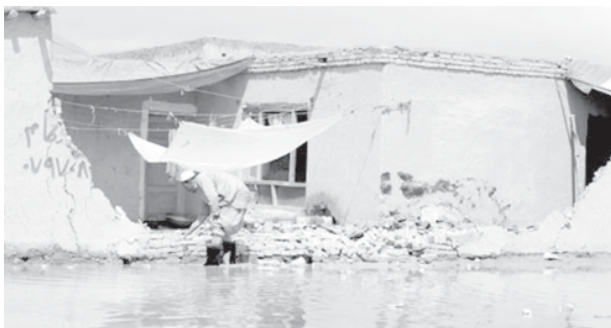
An Afghan inspects his wall damaged by heavy rain in Kabul, Afghanistan, on 2 April, 2009. Heavy rainfall over the past 24 hours in Afghan capital Kabul claimed the life of one young man and destroyed or damaged some mud houses on Thursday. — INTERNET
